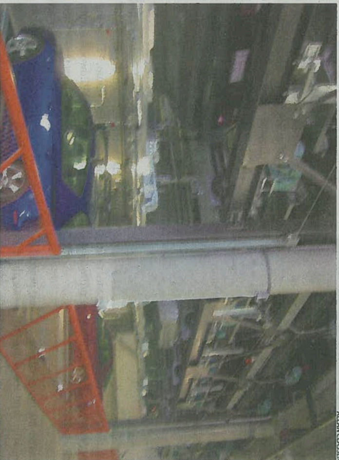
The automated parking system at The Janey can store 25 cars in the floor space of nine. It's the third such system in Portland. All were built by Denver-based Harding Steel.
